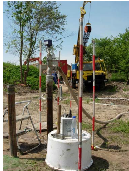
d) 2 inch hose to injection wells
