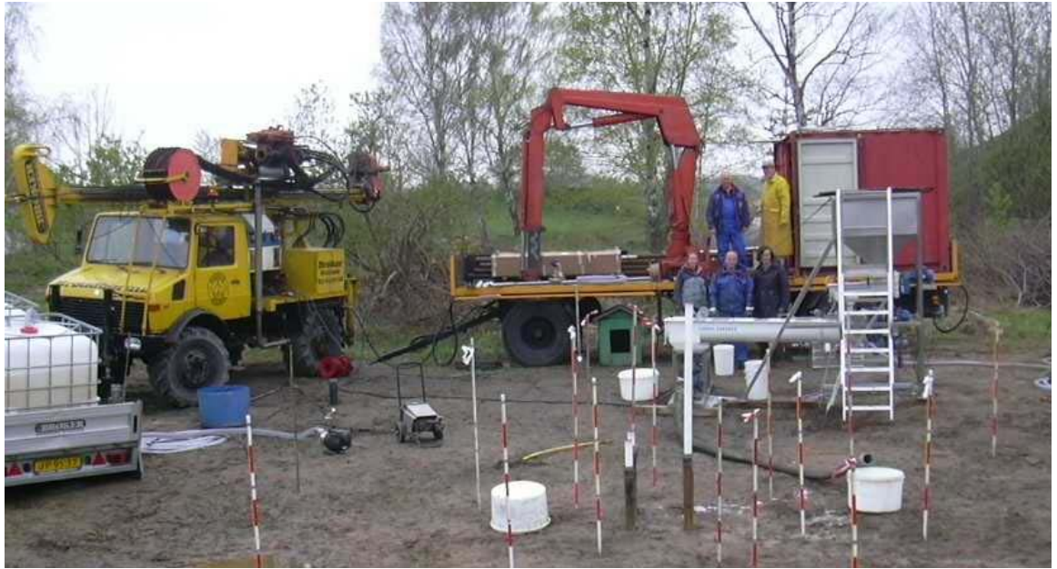
Figure 5. Survey measurements of terrain uplift during injection of hydraulic fractures in the subsurface
